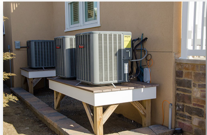
Elevated HVAC units on wooden platform
